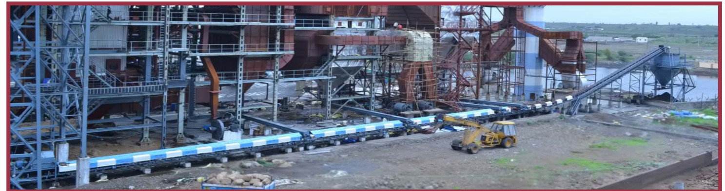
ASH HANDLING SYSTEM
